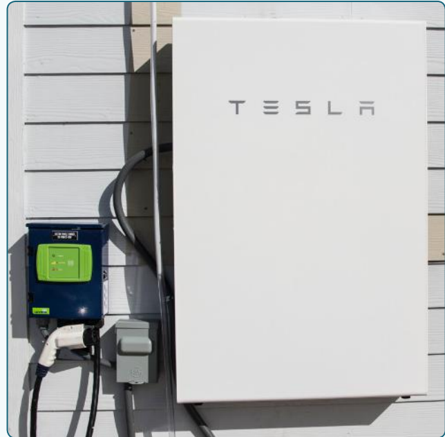
Figure 5: Example of a residential energy storage system with integrated electric vehicle charging, which uses the Powerwall lithium-ion battery made by Tesla, a clean energy industry leader with major manufacturing facilities in Alameda County.
