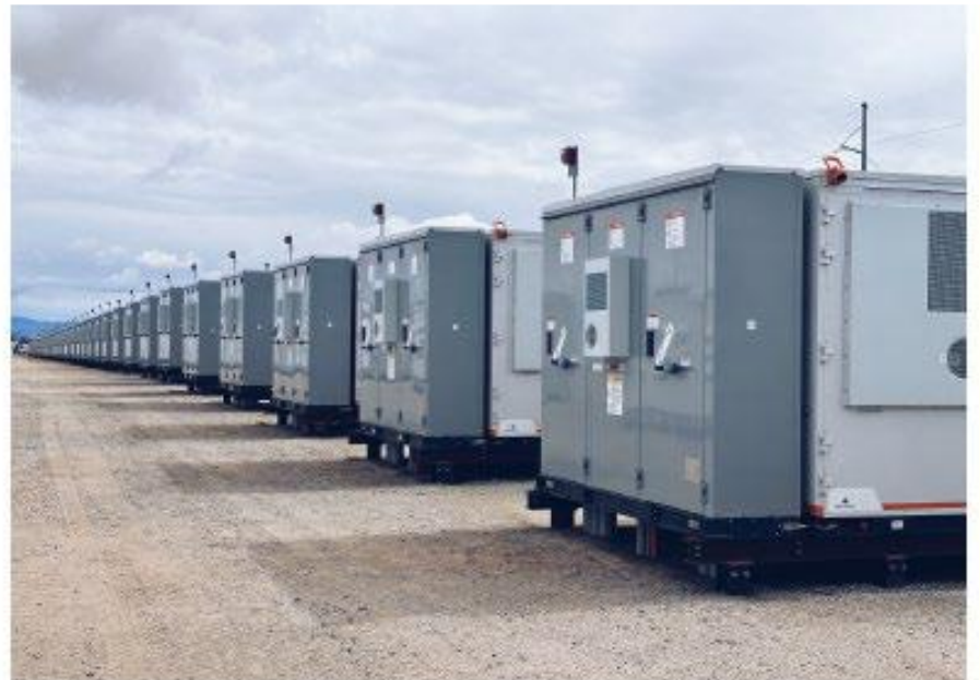
Image Source: Daggett PV+Storage March 2024 Progress Report
