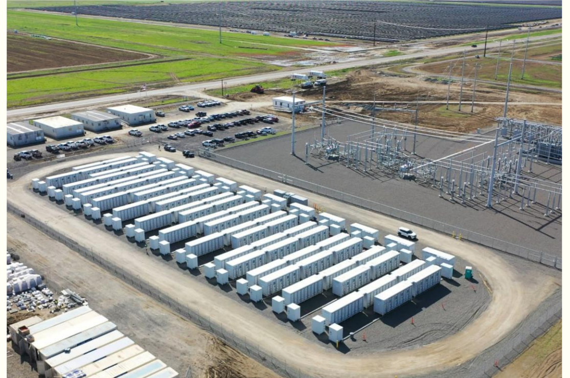
Image Source: Scarlet I PV+Storage Feb 2024 Progress Report
