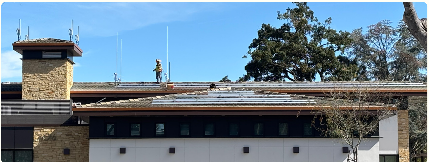
Photovoltaic (PV) solar panels being installed on the roof of the Livermore City Council Chambers.
