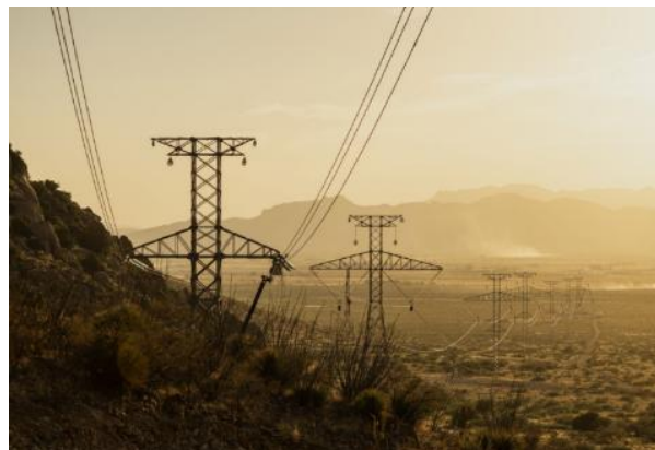
2 Transmission lines connecting to the SunZia project, Central New Mexico
