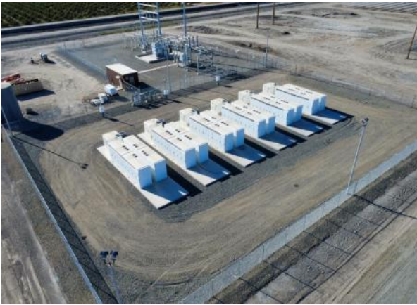
3 Alpaugh Solar Facility, Tulare County CA
